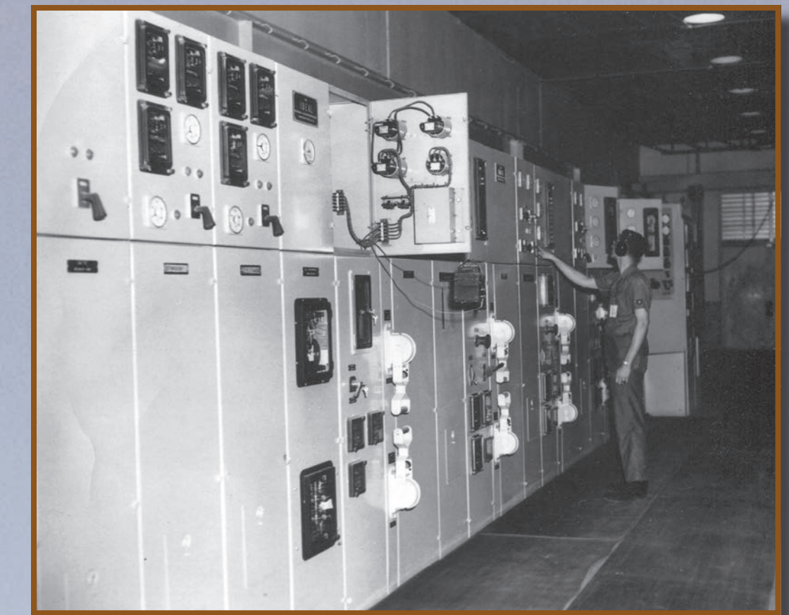
Switchgear inside power plant, operations area, ca. 1960s.
